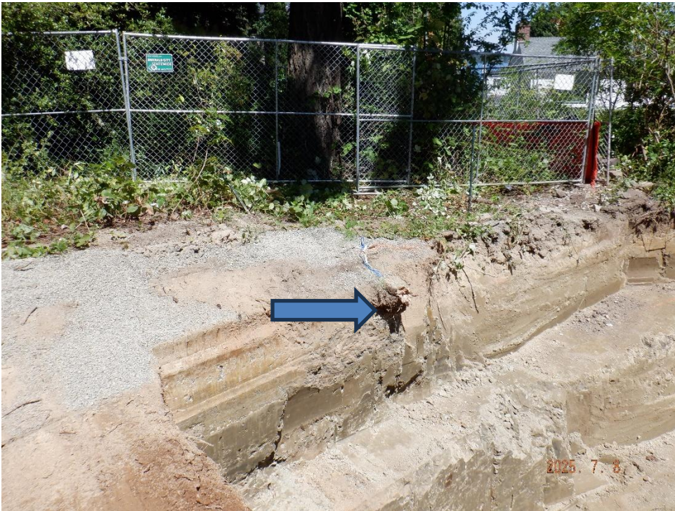
Large structural root exposed at cut bank roughly 18-feet south of Tree #1
