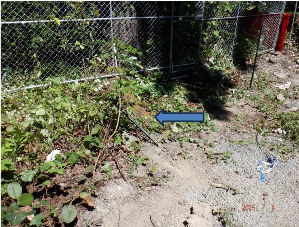
Large structural root needs to be cut at 6-feet from trunk face (at arrow) to accommodate foundation work
